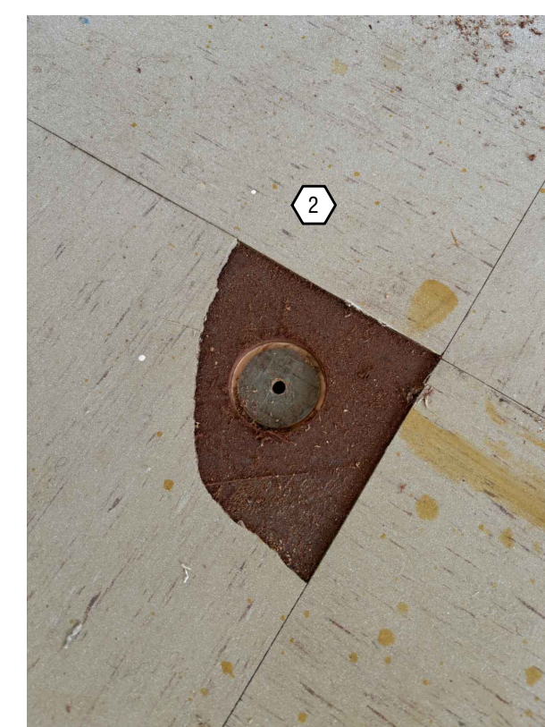
D VIEW OF ACM GRAY MASTIC UNDER VARIOUS FLOORING H100
